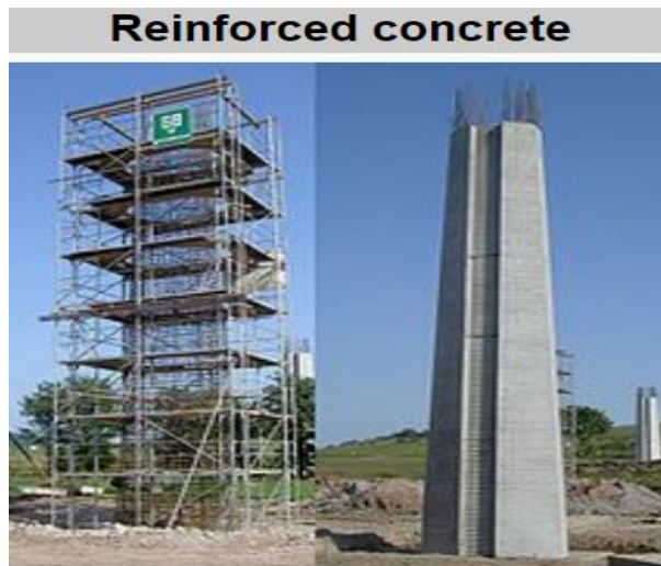
Figure 1: Before and after the concrete was placed in place around the rebar cage of a massive reinforced concrete column
